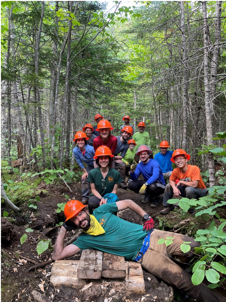
PHOTO: THE CREW PROUDLY SHOWING OFF ONE OF OUR FINISHED BOG BRIDGES
